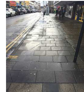
Kings Street's uneven paved area, dangerous? The many repairs and service lids to the paved area in King Street has become a mishmash of surfaces, sizes and uneven heights. This adds difficulty for people with walking difficulties and the blind.
